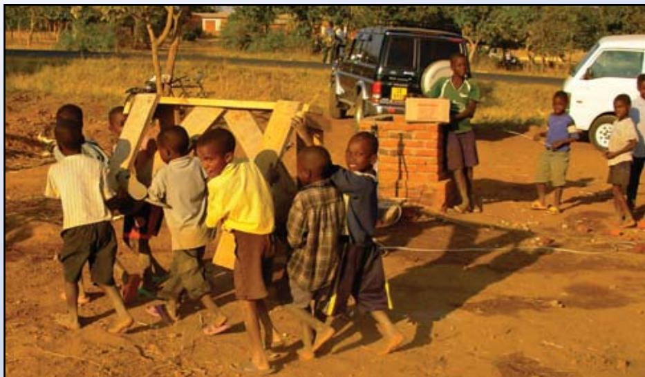
Orphaned boys helping with the construction of the feeding centre in Lumbadzi, Malawi.
