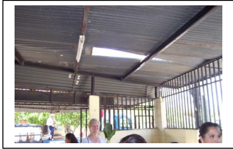
Lorraine standing under the hole in the roof.
